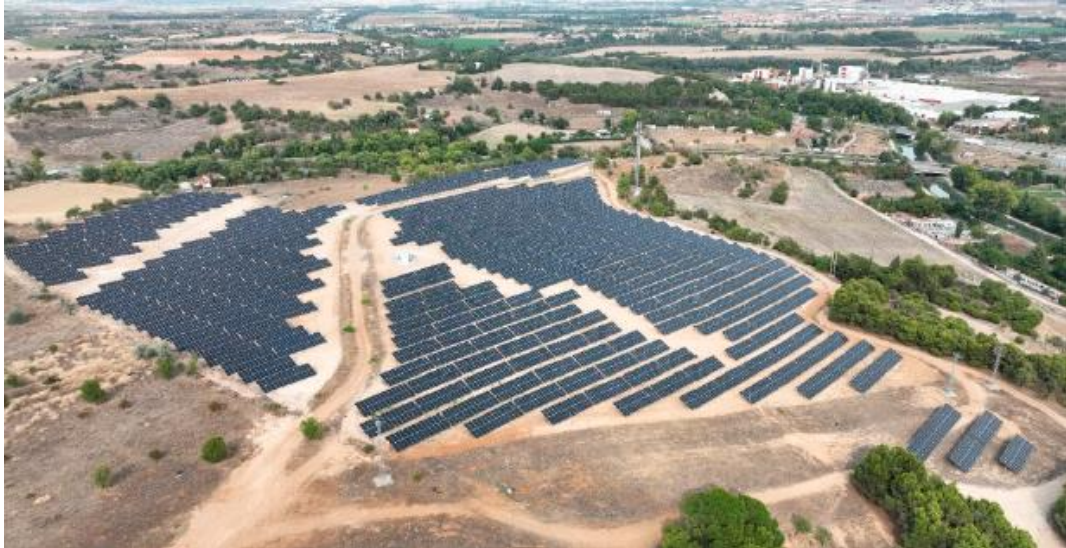
Ground-mounted photovoltaic installation for industrial self-consumption for Lingotes Espaciales SA. Power of 5.9 MW in Castilla y León.
